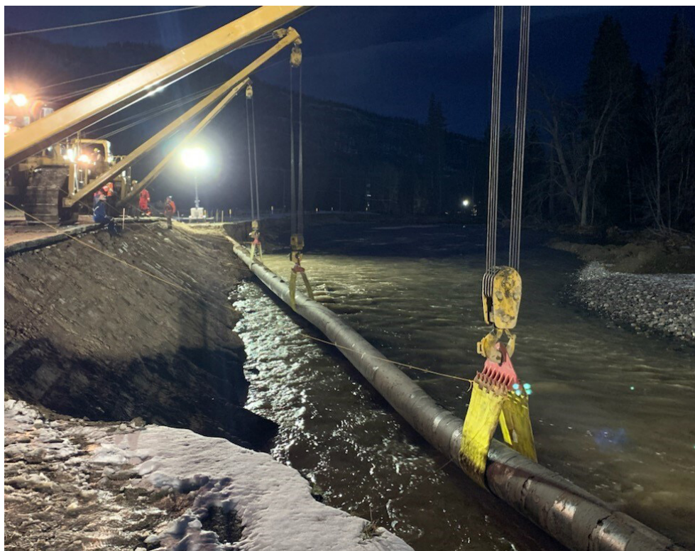
Figure 5. Sidebooms supporting pipe in the Coldwater area.
